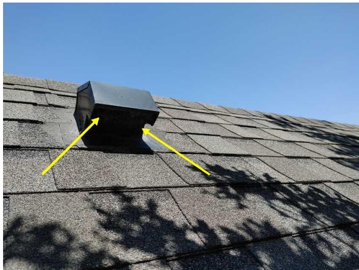
Screened dryer vent full of lint at roof peak
