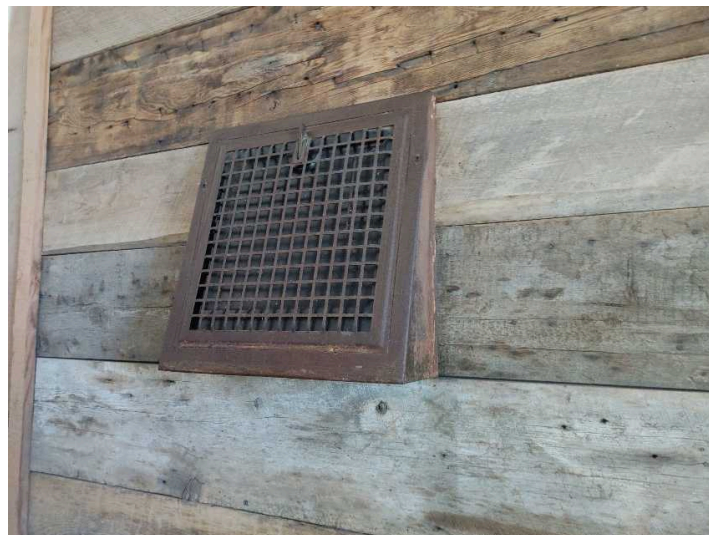
Missing venthood at kitchen cook top
