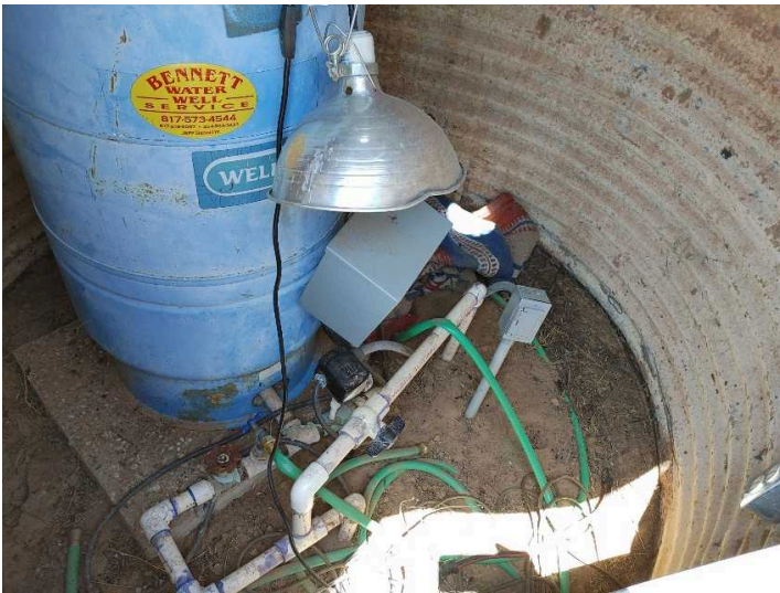
Pressure tank appears adequate
