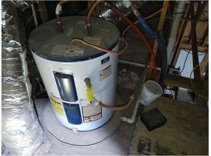
Older electric water heater unit located at garage-barn location
