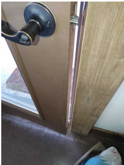
Side entrance door catches at threshold
