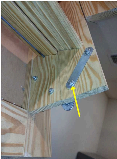
Loose hardware bolts
