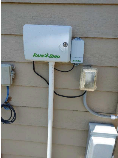
Lawn irrigation equipment performed adequately
