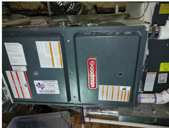
Furnace to main structure is LP Gas
