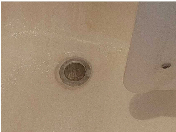
Missing drain stop at tub basin
