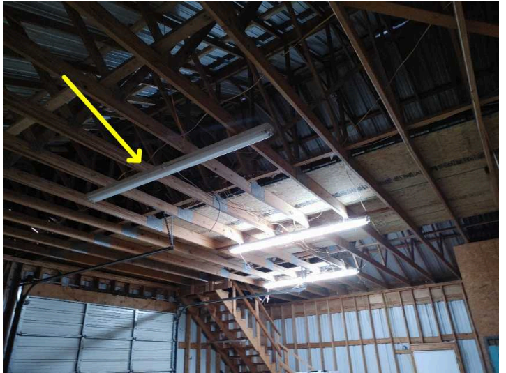
Fluorescent light fixture(s) inoperative at garage
