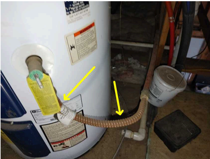
TPRV reduced in size at the 38 gallon water heater unit
