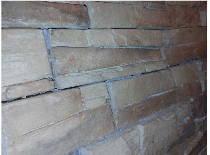
Grout deterioration between stones inside shower enclosure
