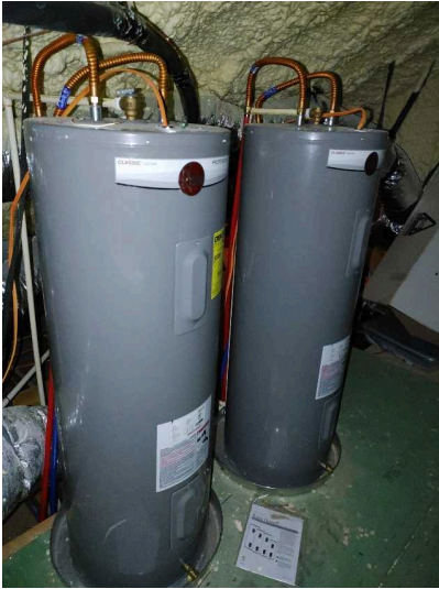
2-50 Gallon Electric Water Heater Units located in attic
