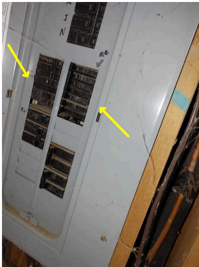
Service main in garage missing labeling identification
