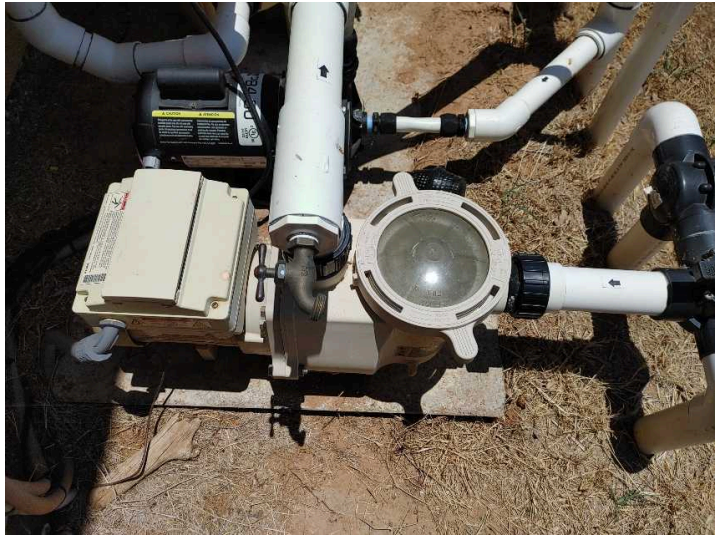
Variable speed pump motor and skimmer performing adequately
