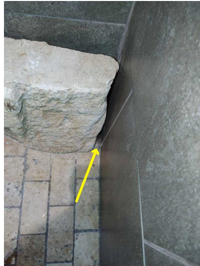
Openings around shower enclosure
