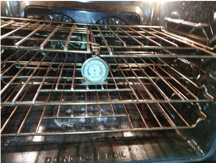
Top oven heating adequately
