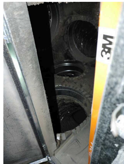
Duct cleaning advised at main structure
