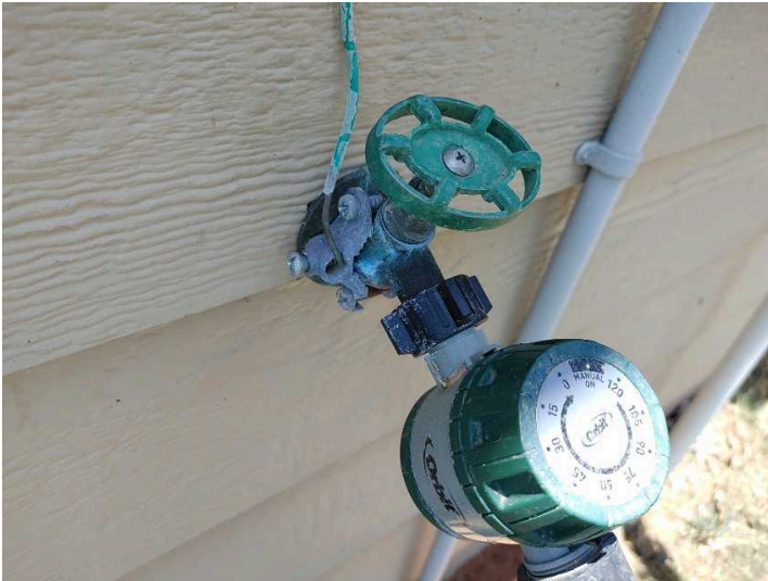
Missing backflow devices at exterior hosebibs
