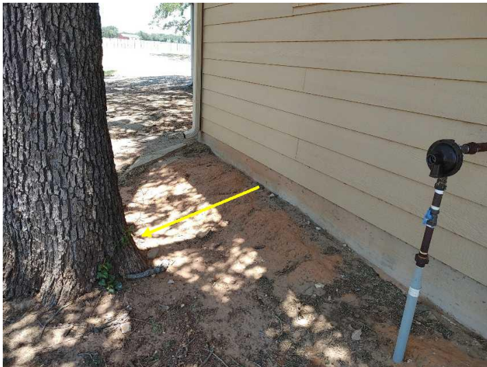
Large tree growing within 10 feet of structure
