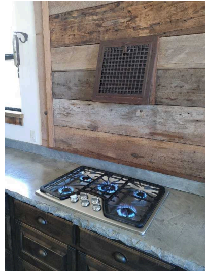
Gas fired appliances should have a method to vent out exhaust
