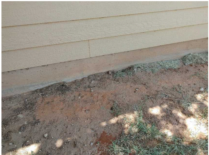
Dry soils around foundation should be hydrated
