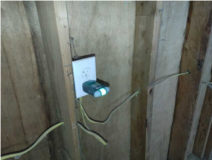
Electrical outlets in garage should be GFCI protected for safety reasons
