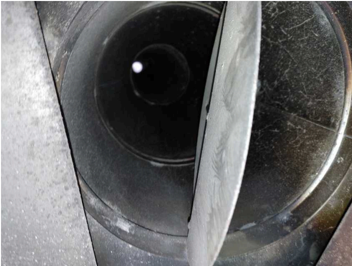
Flue to outdoor chimney appears adequate
