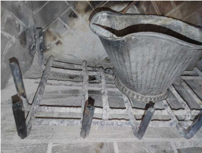
Outdoor fireplace appears adequate
