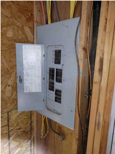
Service panel #2 located at garage-barn location (Adequate)
