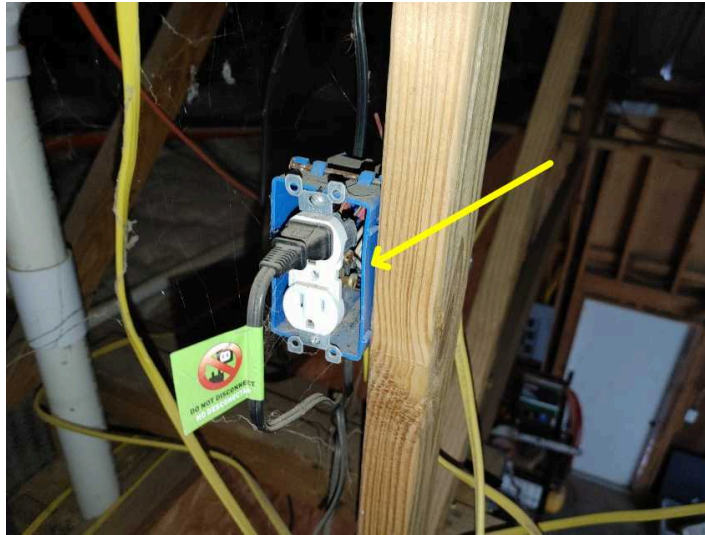
Various plug outlet covers missing at garage-barn location(s)
