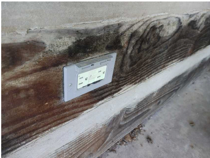
Missing cover-plates at exterior plug outlet
