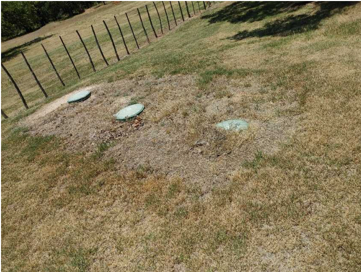
Septic tank situated rear of structure at south side property
