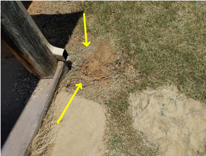
Missing splash-blocks and/or underground drainage system
