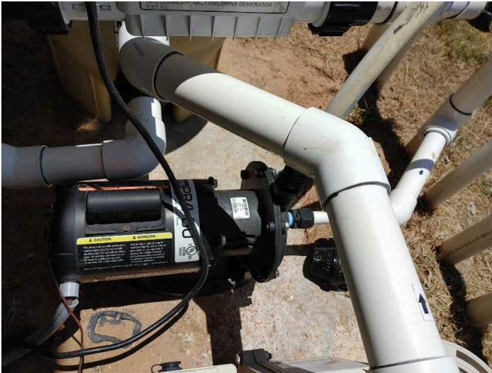
Booster pump performing adequately
