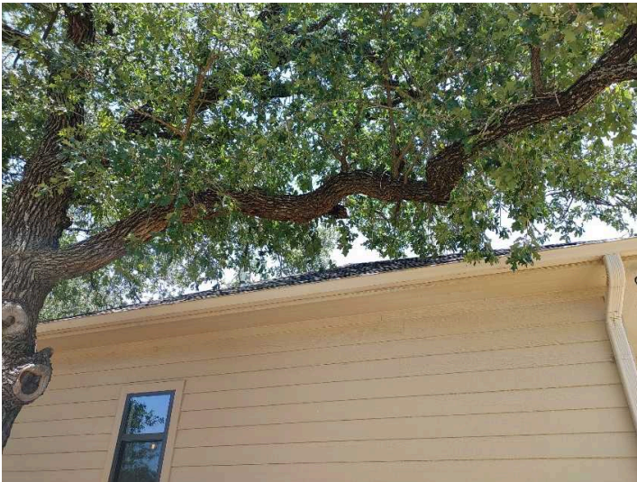
Tree limbs in contact with roof deck
