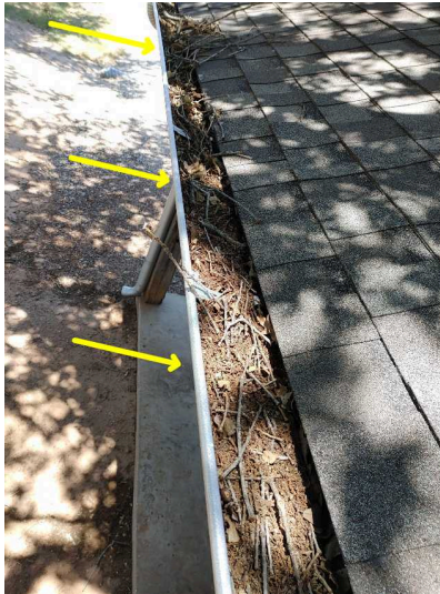
Rain gutters full of tree limbs and debris
