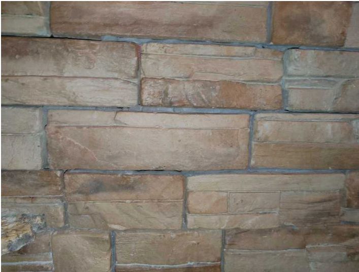
Various stones appeared loose at interior shower enclosure
