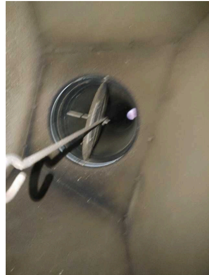
Creosote should be cleaned from chimney before further usage
