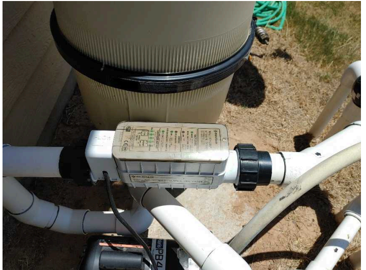
Salt-cell/Chlorinator appears to be performing adequately
