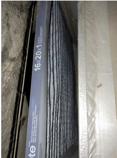
Filter replacement advised at the garage-barn location
