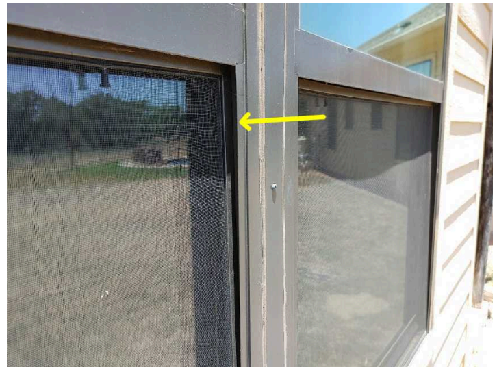
Loose or damaged screens at various exterior location(s)
