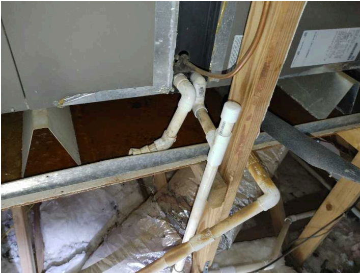
Shutoff sensor should be applied to the condensate pan or at the backup drain
