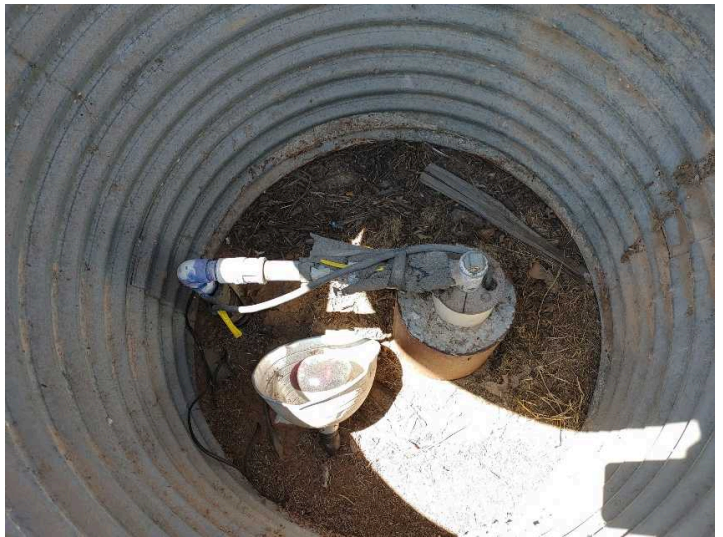
Drilled well and sanitary cap located at front of property
