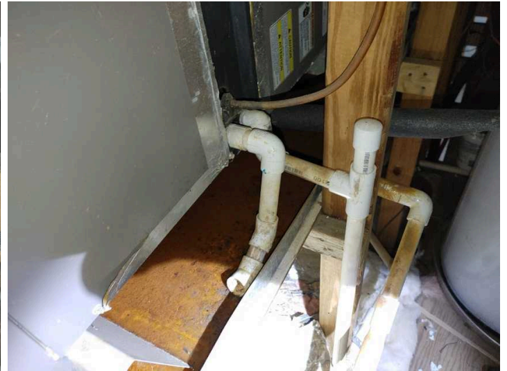
Standing water and rust in the drip pan should be cleaned before further usage
