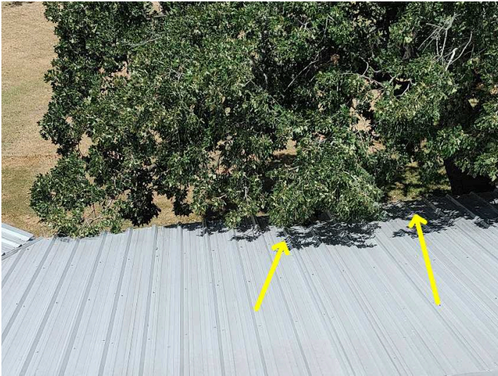
Tree limbs in contact with metal porch awning should be trimmed back minimum 6' from the covering
