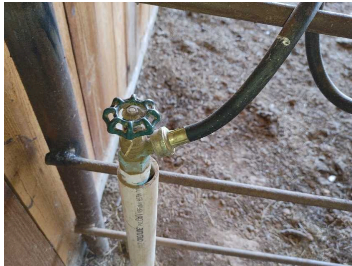
Backflow prevention advised at each exterior hosebib
