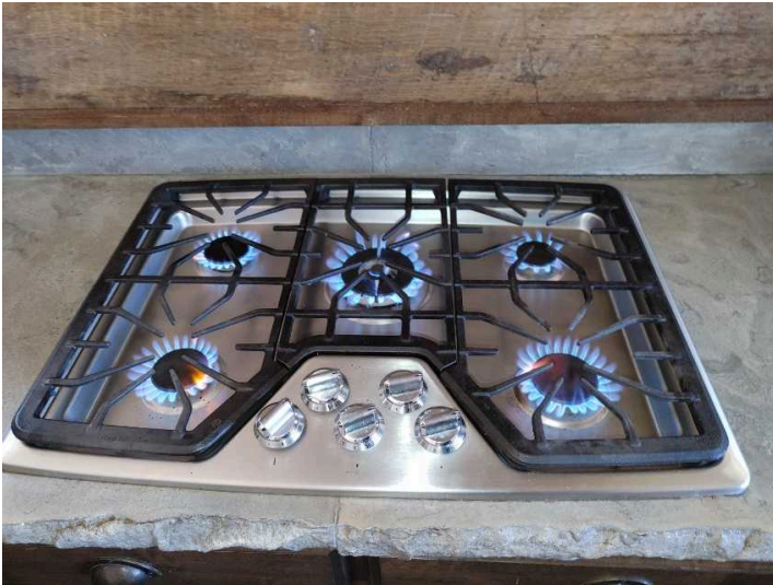
LP Gas cook top appears to be performing adequately
