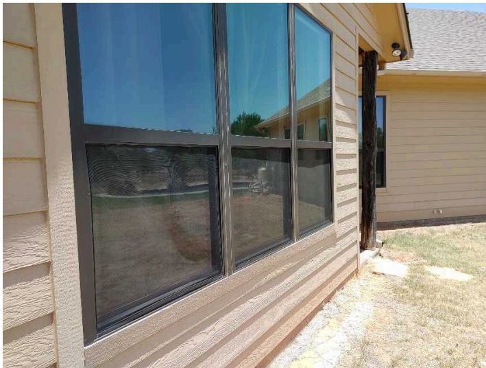
Lost seal(s) between glazing may occur during temperature changes
