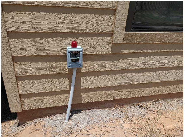
Septic alarm appears adequate
