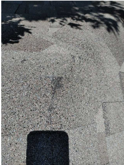
Fiberglass strand exposure at end of peak(s)
