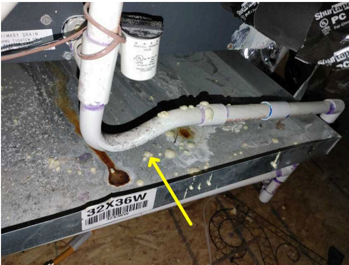
Insulation tubing should be applied around primary drain to prevent condensate blockage
