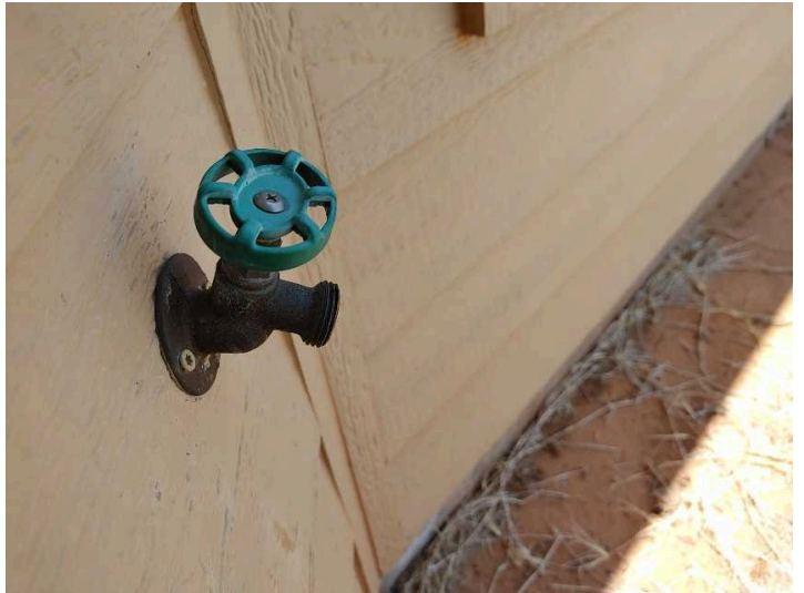
Backflow prevention advised at exterior hosebib
