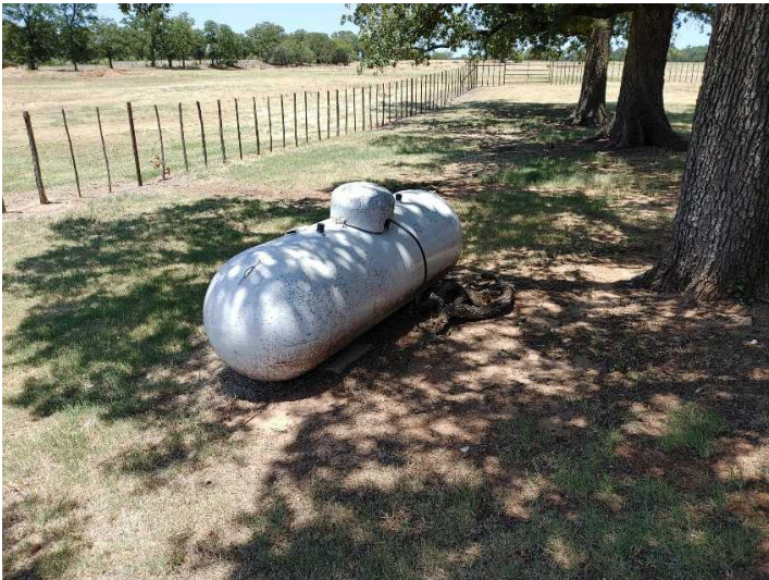
Propane storage tank located NW of structure
