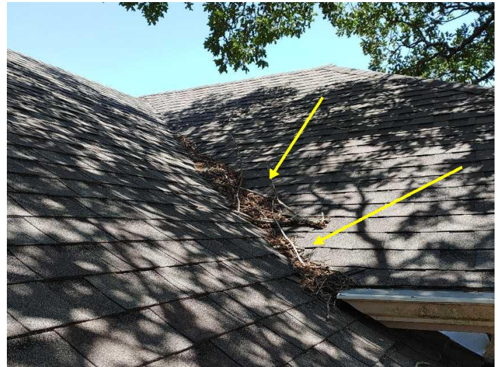
High foliage near roof should be trimmed back
