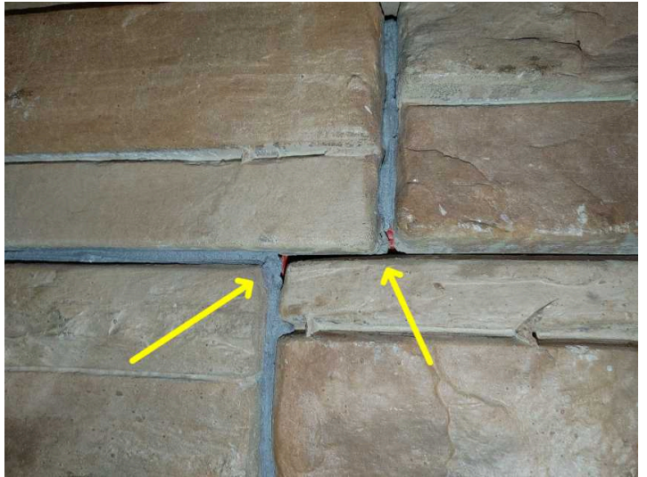
Openings in grout seams between stones at main shower enclosure
