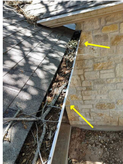
Rain gutters should be kept clear at carport
