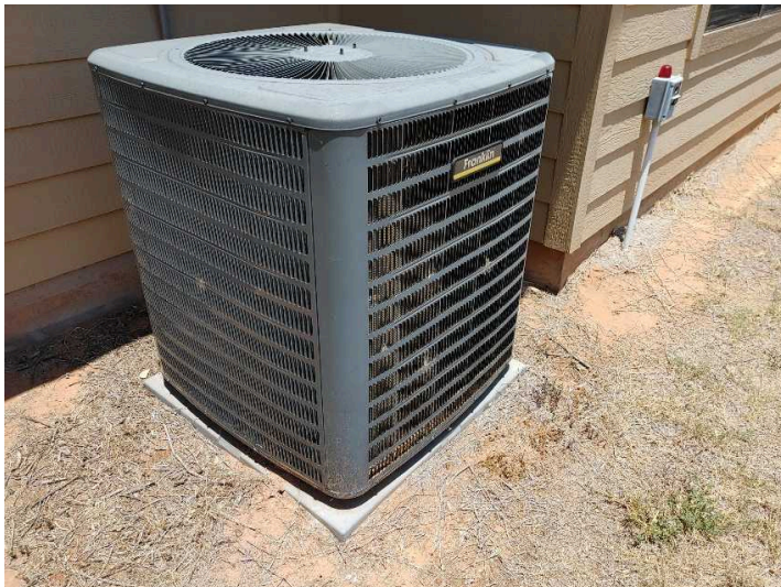
Outdoor condenser-unit located at rear of main structure
