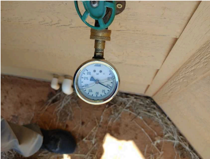
Static water appears adequate
